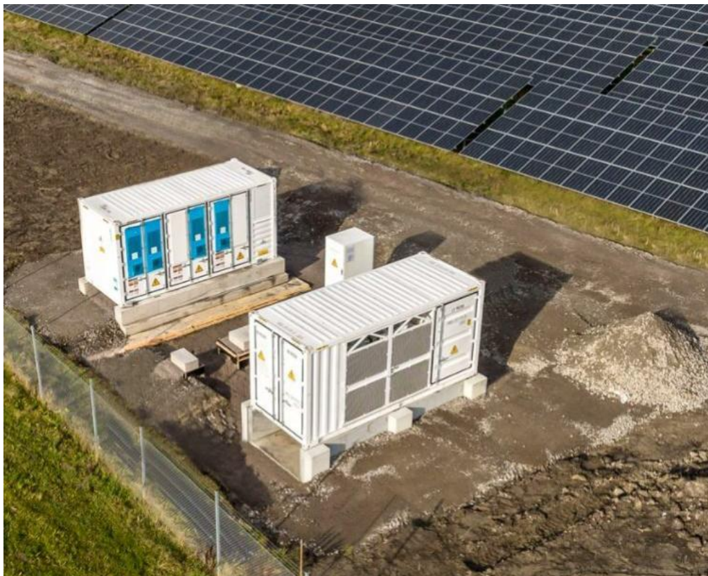
Figur 6. Batterilager, container-baserad lösning.
